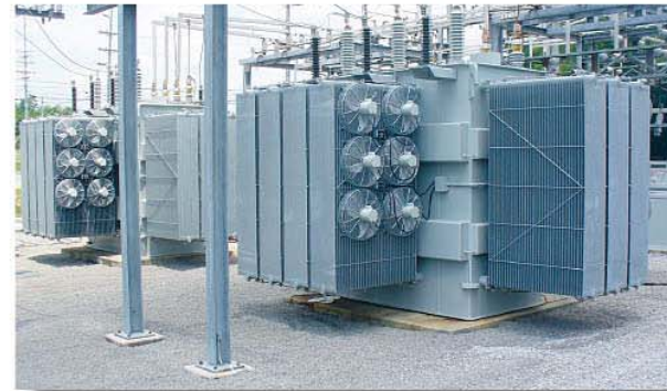
New transformers which doubled the capacity of the Lantana Substation in Cumberland County were installed in 2013.
