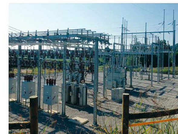
The new Byrdstown Substation that served Pickett County was completed in 2012.
