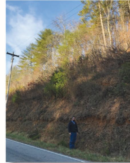
Aaron Hood, Working Sub-Forman Benton Service Area, stands beside the embankment to give height perspective.
