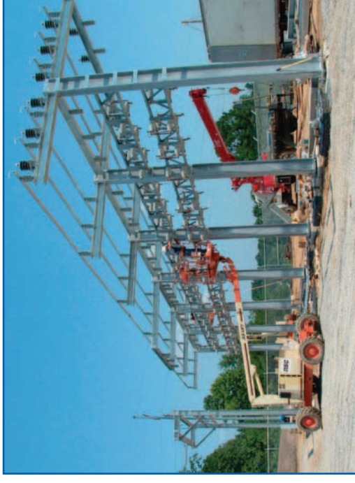
Volunteer Energy Cooperative crews, as well as contract crews, are completing major renovations at the Hopewell Substation on Rabbit Valley Road in northwest Bradley County.
