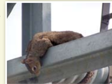
This squirrel caused extensive damage to a main substation breaker and created a power outage that affected about 1,200 VEC member/owners.
