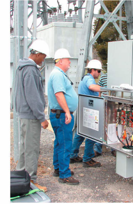
Bill Ntwali, left of DCI, the company providing AMR components to VEC, and Darrell Crisp, VEC's superintendent of metering and substations oversee crews as they activate automated metering at the Ten Mile Substation.
