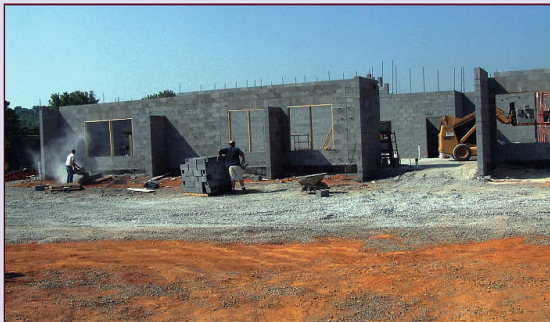
Work is proceeding on Volunteer Energy Cooperative's new Spring City Customer Service Center which is scheduled to open for business this fall.
