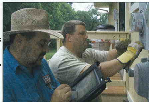
Morris Swafford, left, and Courtney Gregory install Automated Meter Reading (AMR) equipment at the home of a VEC customer.
