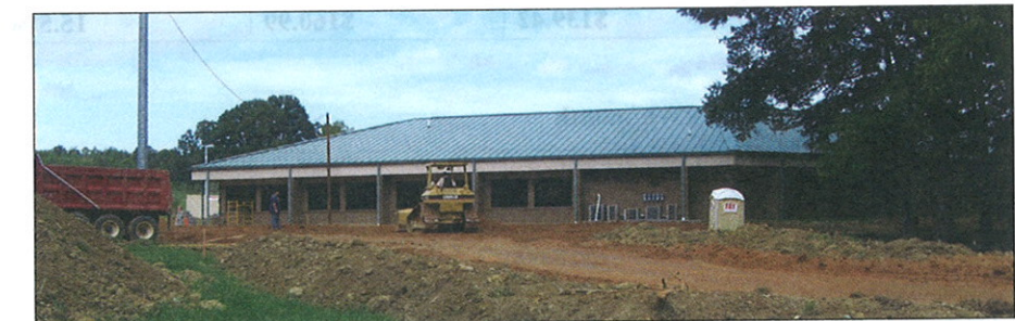
Construction is under way on VEC's new centralized dispatch call center at the Corporate Offices in Decatur. The new call center will allow us to centralize and streamline our outage response and many customer service functions.
