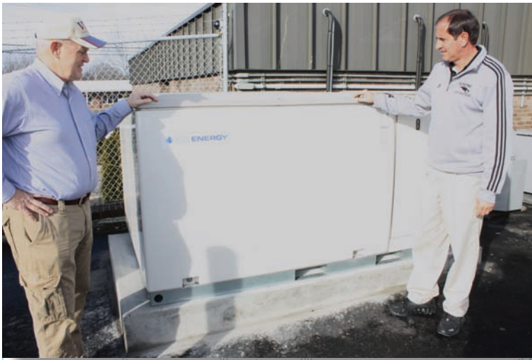
The Ice Bear units that were recently installed at VEC's Jamestown and Monterey offices look very similar to a traditional central air conditioning unit – but they operate very differently.
