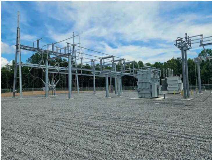
Pleasant Grove Substation
