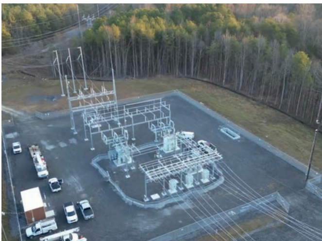
Pleasant Grove Substation Drone View
